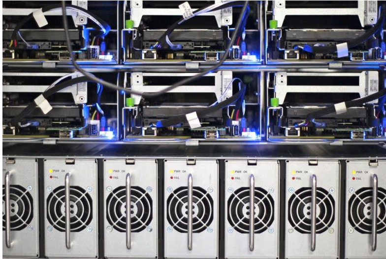
Figura 15: Micro servidor Open Compute Project
